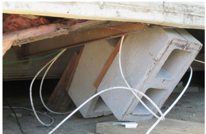
Manufactured home rotated and fallen support piers.
