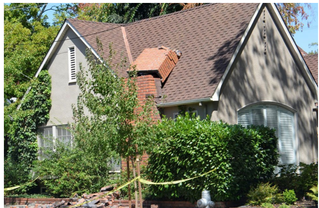
Earthquake damaged chimney.
